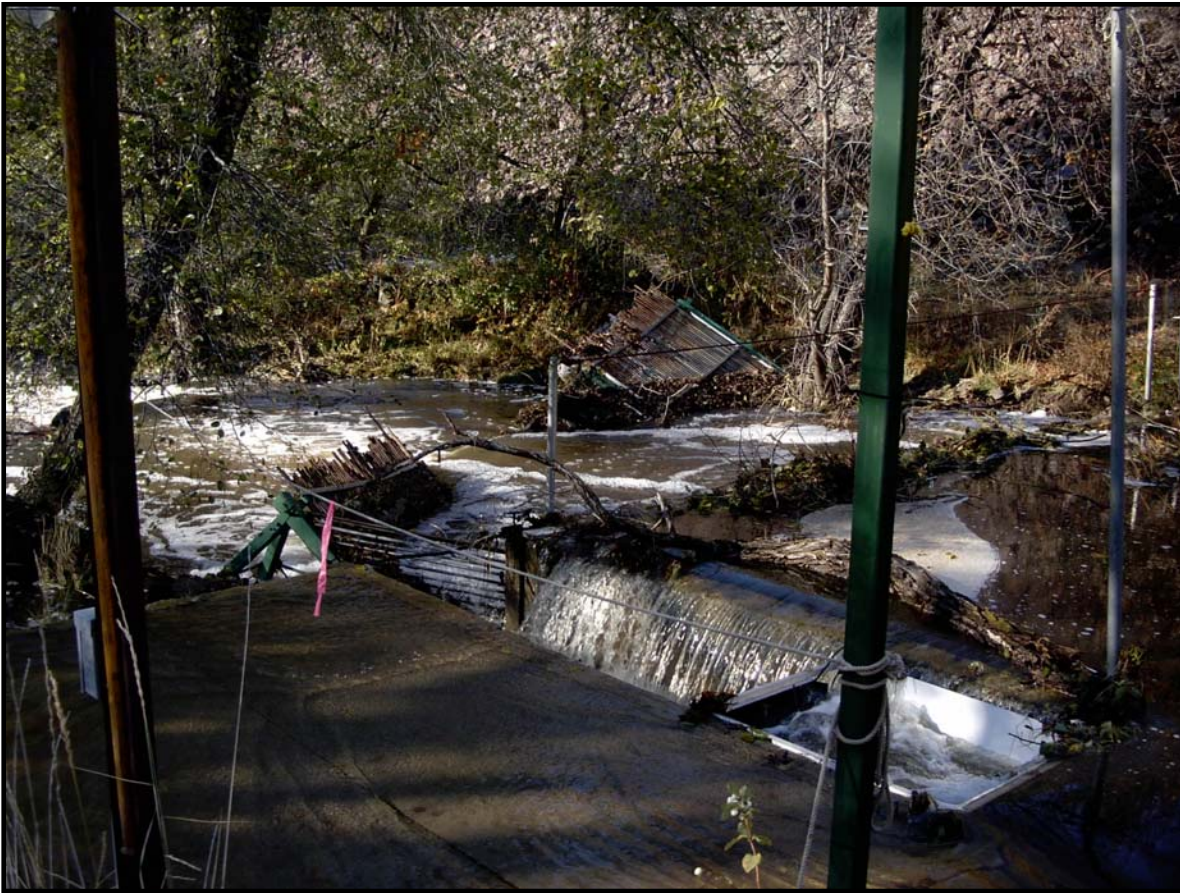
Figure 3. Photograph of the BCFCF taken on November 8 th after peak flows had receded. The damaged camera housing (lid removed) is visible in the lower right corner. The collapsed tripods are visible in the left center of the picture downstream of concrete raceway and pad.
