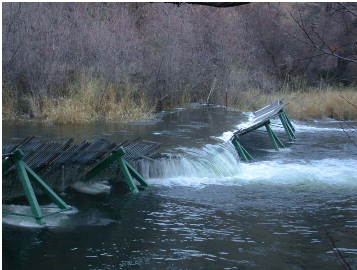
Figure 14. Ice buildup caused the collapse of a tripod supporting the Alaskan weir at the SRFCF, December, 4, 2009.
